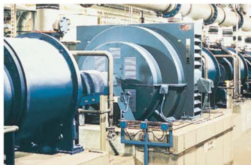
Synchronous motor 1750 HP at 240 RPM with Paper Mill Dripproof™ enclosure and double shaft extensions driving vacuum pumps in a paper mill.
