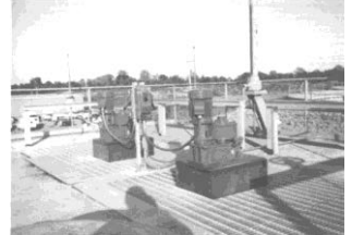
Paramax Reducer used for sawmill drive.
