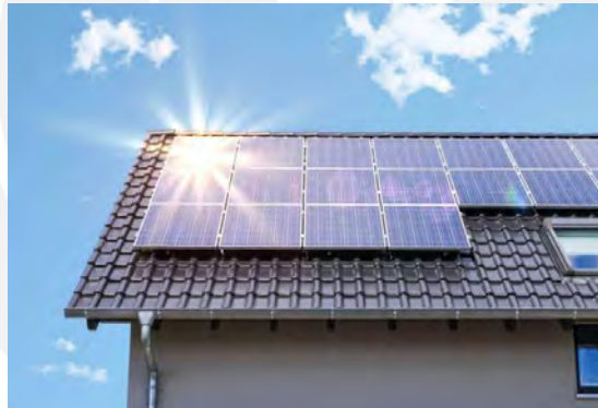
Figure 9: Residential PV system.
