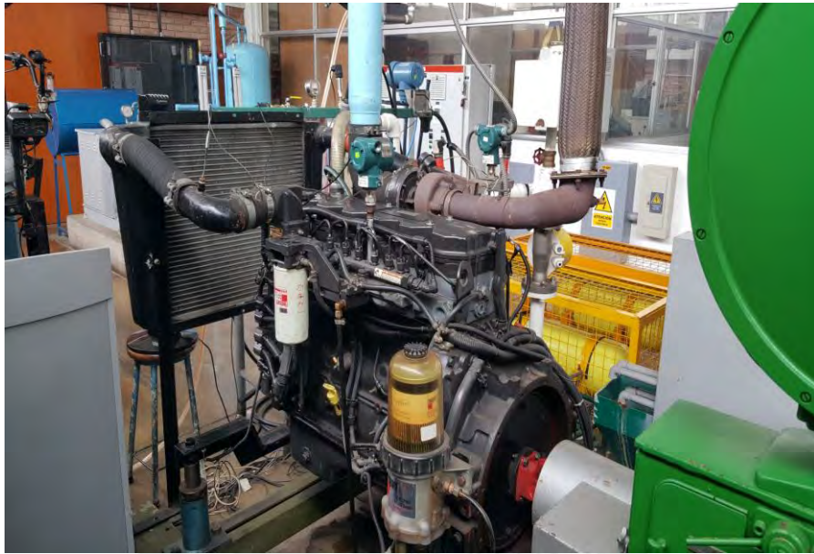
Figure 3.14: Diesel engine for analysis (Energy Laboratory, PUCP)
