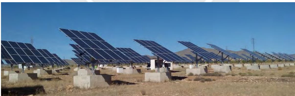
Figure 5. PV generator located in Granada, Spain [50]
