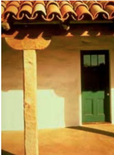
Figure 29. Tapered barrel clay roof tiles custom made for the restoration of the 1820s “Indian barracks” at Mission Santa Cruz in California. Photograph by the National Park Service 18 (Grimmer & Williams, 1993, p. 1)
