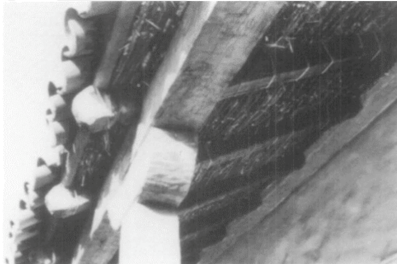
Figure 36. The underside of a roof on the restored barracks at Santa Cruz Mission showing the twig sheathing to which the clay tiles were attached with mud mortar.
