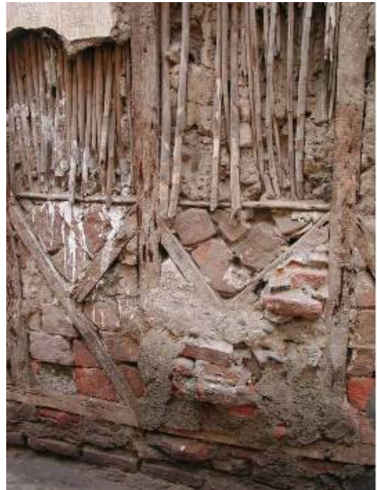
Loss of rigidity by damages in wall foundation
