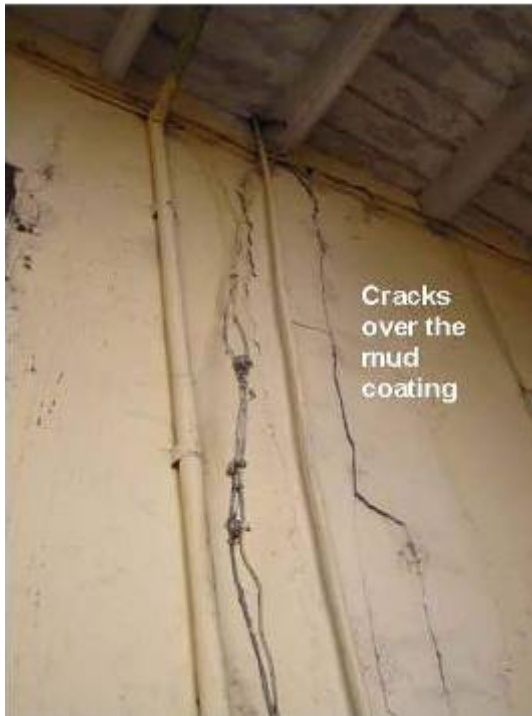
Cracks on mud coating
