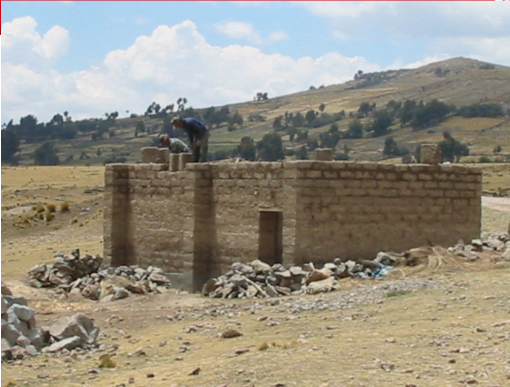
Seismic strengthening of new construction: provides anchorage by extensions to adobe walls
