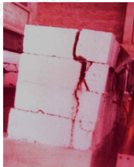
Collapse by tumble effects (photograph by San Bartolome)
