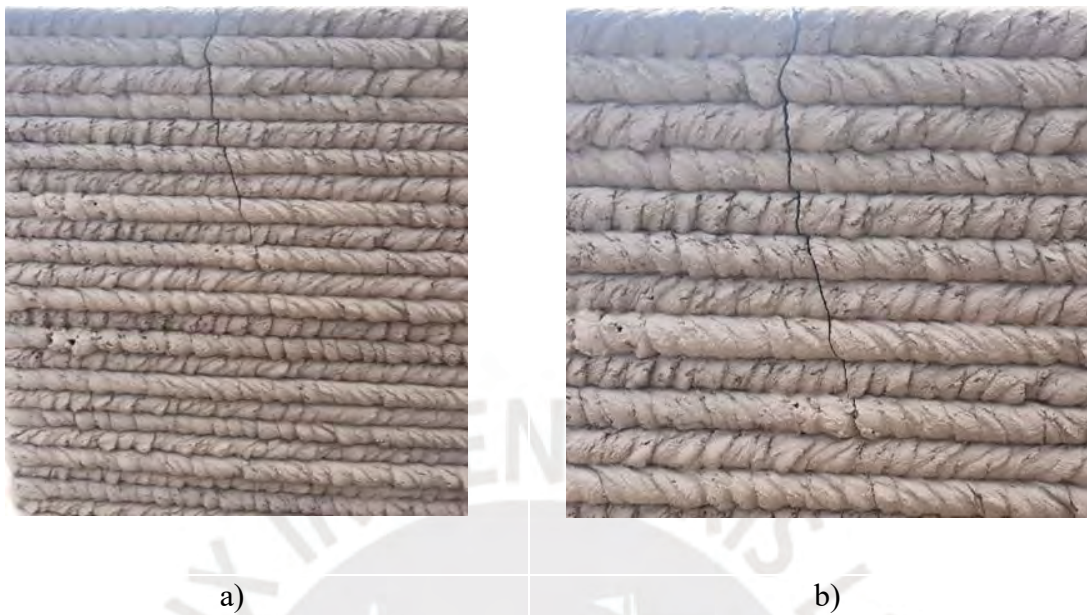
Figure 4.14. a) Fissure in a soil-cement mix until the eleventh layer downwards, b) Zoom of the fissure.
