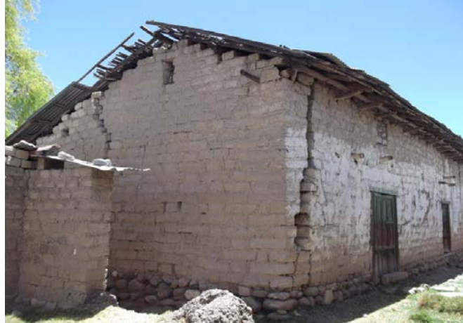
Figure 2. Inhabited damaged adobe house.
