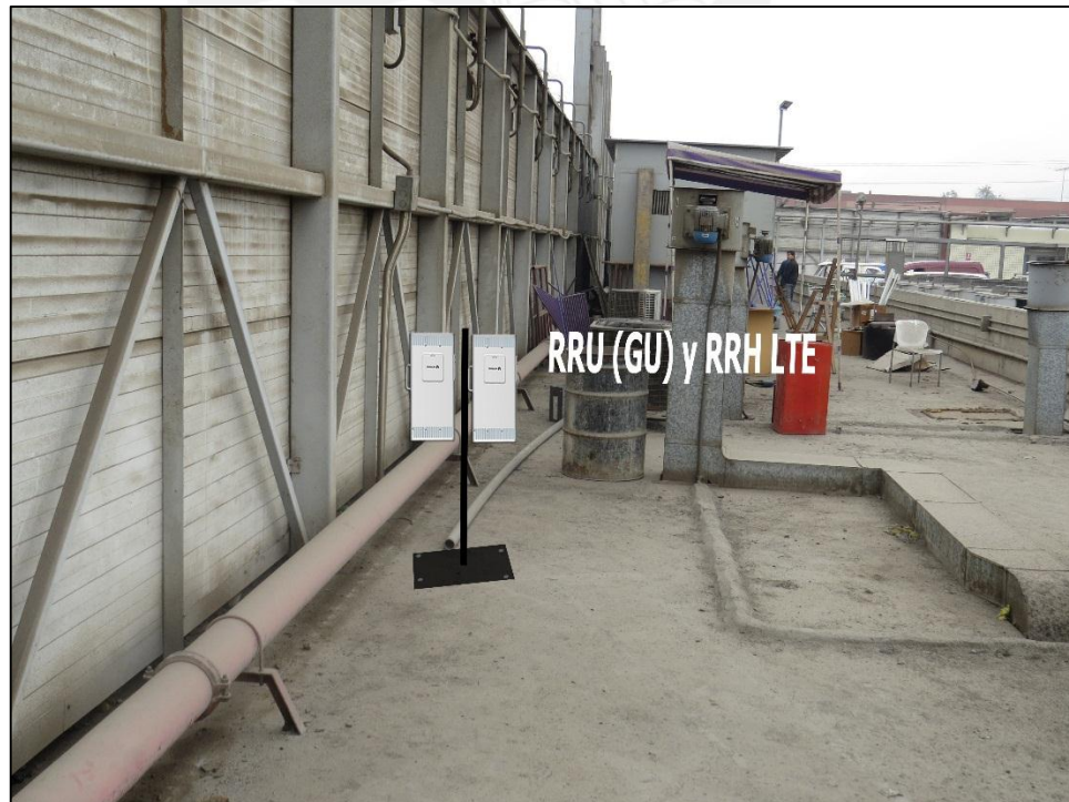
FIGURA 1-3: RRU y RRH DE SECTOR 2
