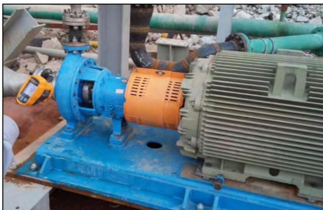
Figura 4.19 Bomba Horizontal de Pit Dewatering
