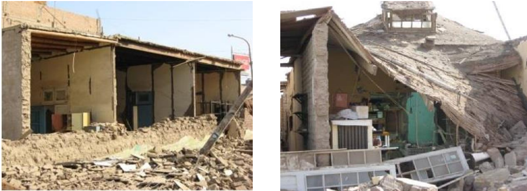
Fig 1. Collapse of façade walls of adobe houses due to the Pisco (Peru) earthquake of 2007
